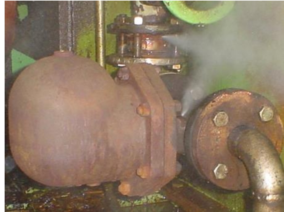
閥件外殼穿孔洩漏
